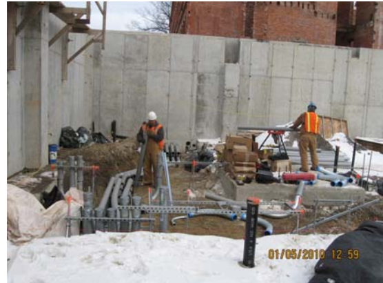
DUGGAN SCHOOL - electrical room underground
